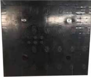
Pict.1) OUTER VIEW OF THE PANEL
